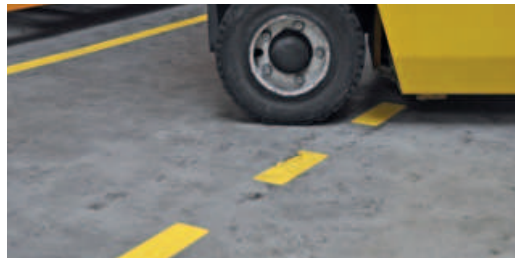
Damage only to individual segments
